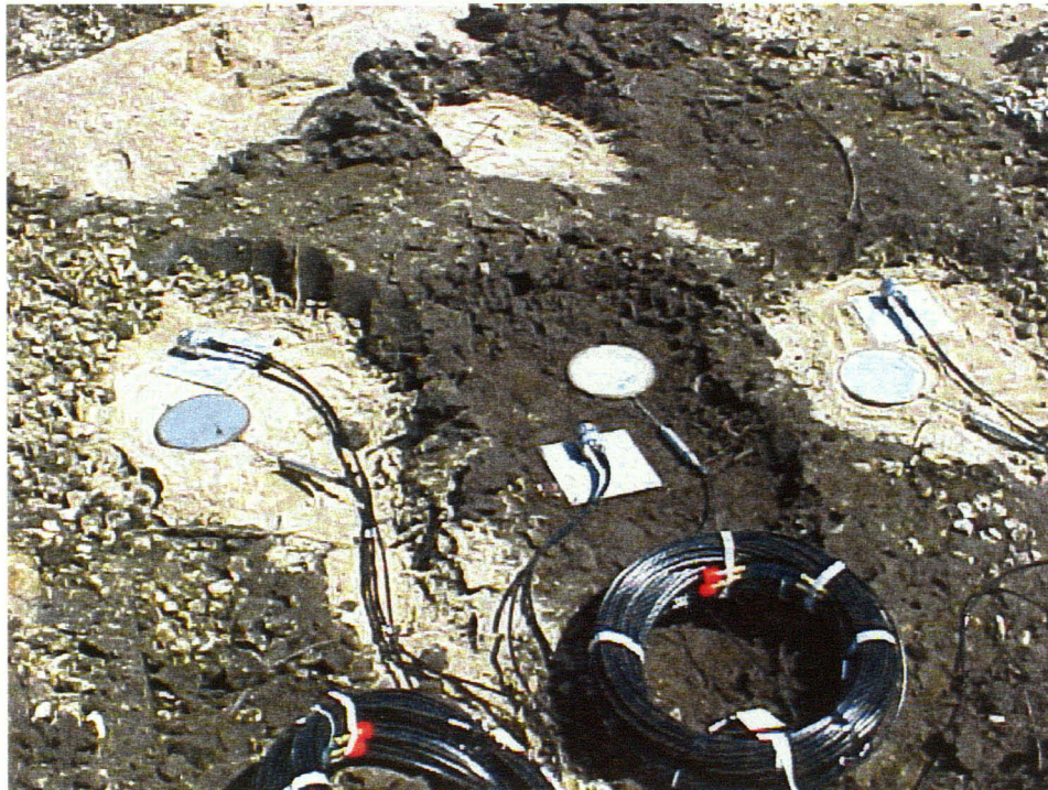
Figure 39. Settlement cells and total stress cells at Ramp "C"
